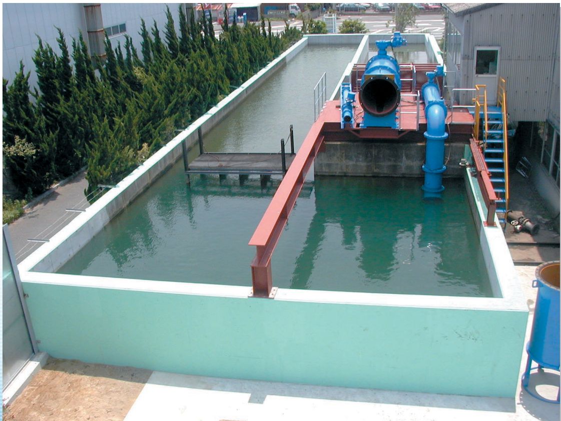
Large Water Tank for Large Sized Pumps
